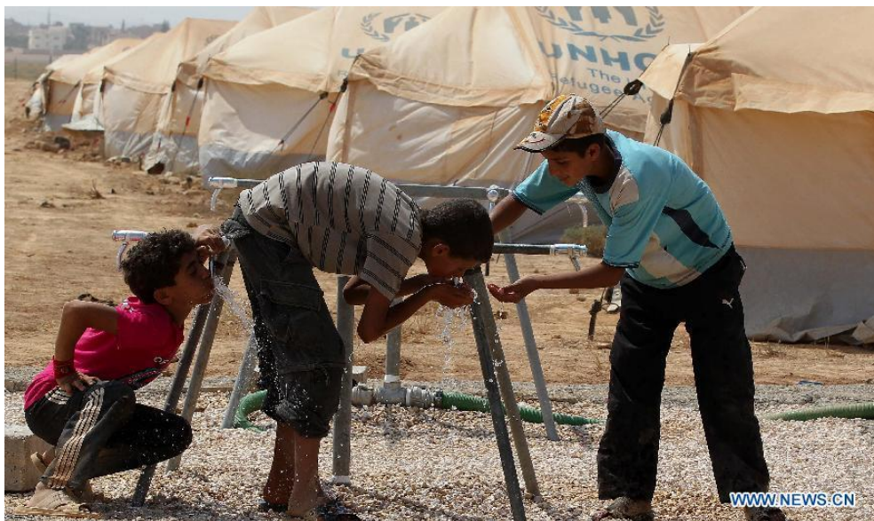
Plate 15 - Water tap in Zaatari camp (source: Unicef)
