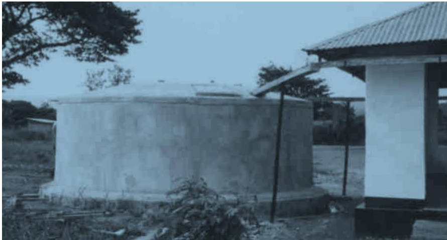
Plate 5 - Example of rainwater harvesting roof system in Rwanda (Source: Practical Action, 2008)
